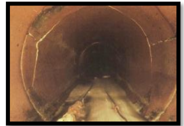
Cracked Clay Sewer Pipe
