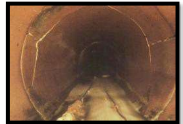
Cracked Clay Sewer Pipe
