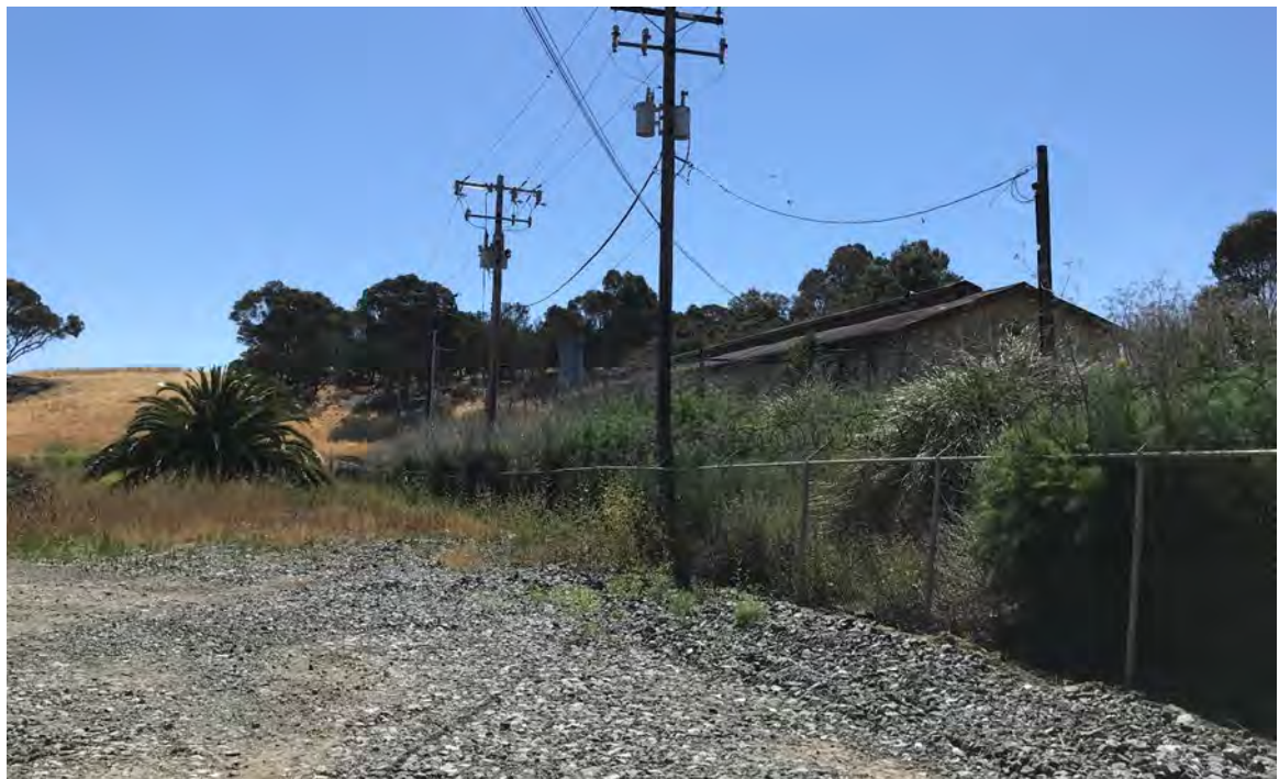
Photo 8. View along the southern FERRF boundary landfill gas collection and control system flare and building within Bedwell Bayfront Park.
