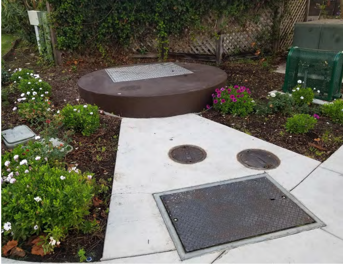
Photo 21. Example of an IPS wet well. Note: the diameter of the wet well shown above is 6-feet in diameter. The proposed wet well would measure 12-feet in diameter.
