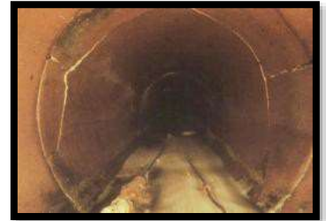
Cracked Clay Sewer Pipe
