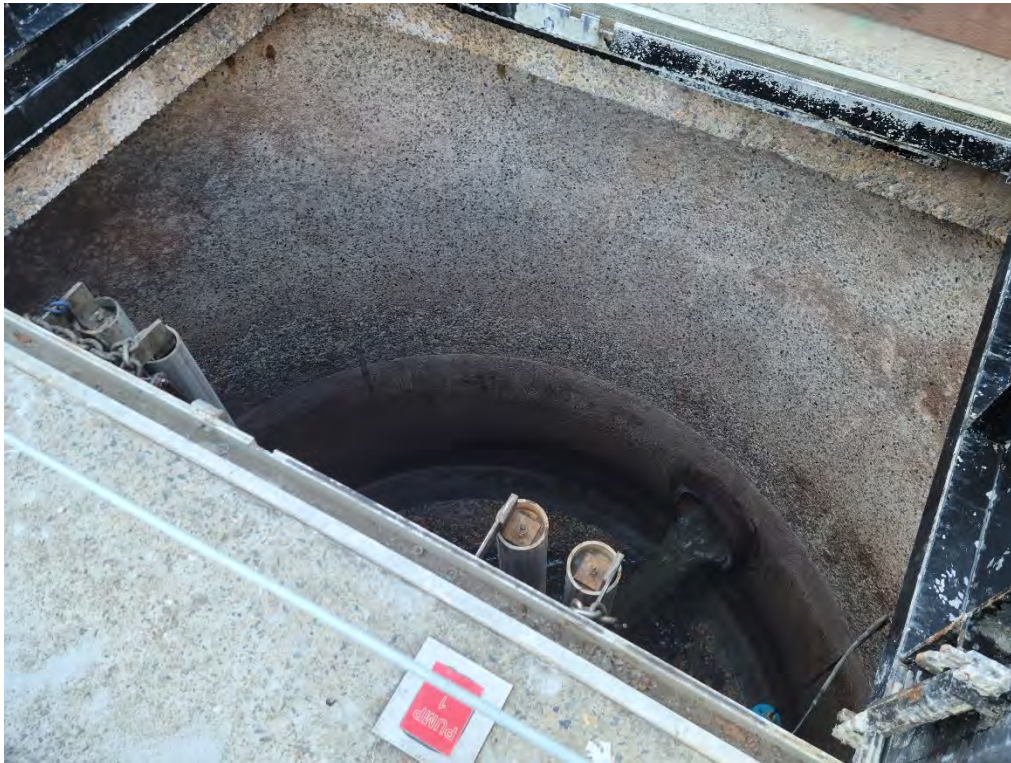
Figure 3 - Wet Well Corrosion Above Water Surface at Hamilton-Henderson Wet Well Walls
