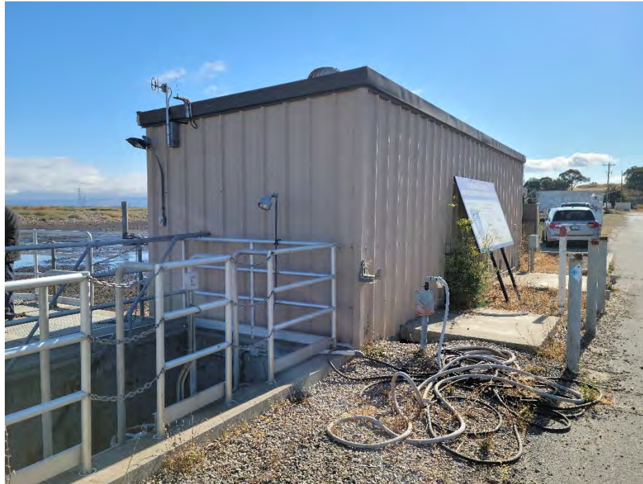
Figure 4 - FERRF Pump Station
