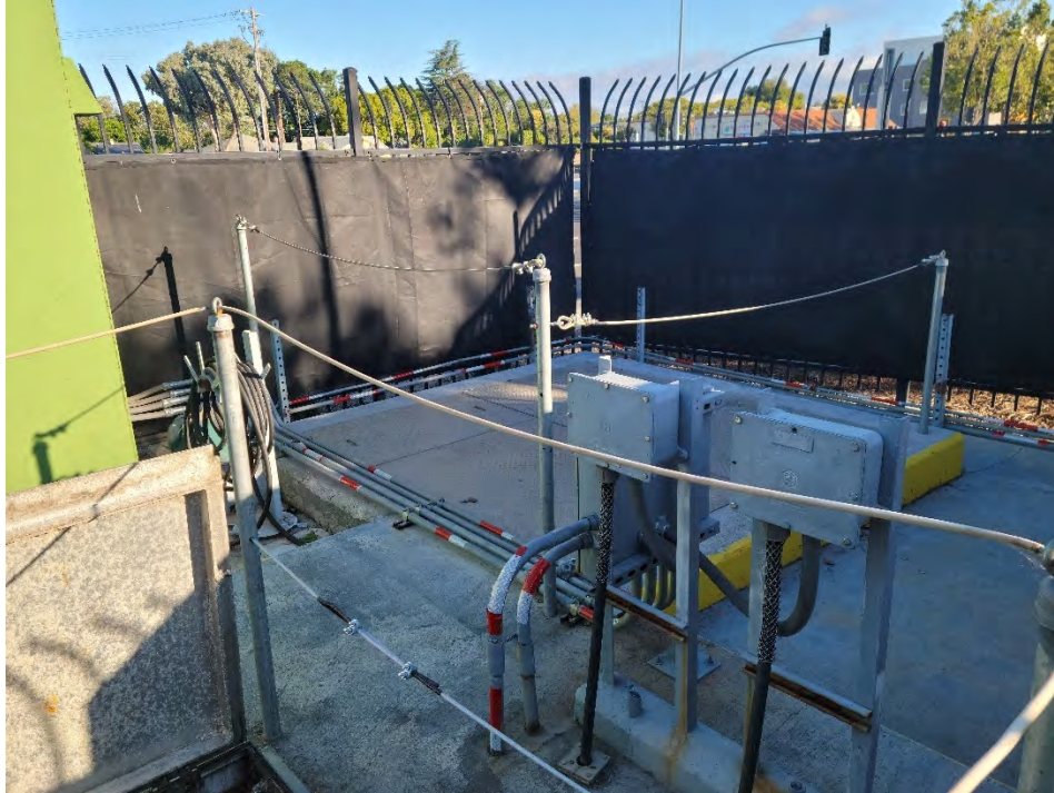
Figure 1 - Willow Pump Station Wet Well Cover and Equipment
