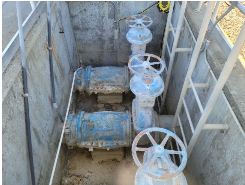
Figure 7.5 FERRF Pump Discharge Valves
