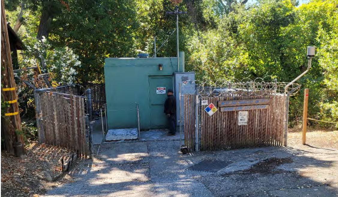
Figure 2 - Stowe Lane Pump Station
