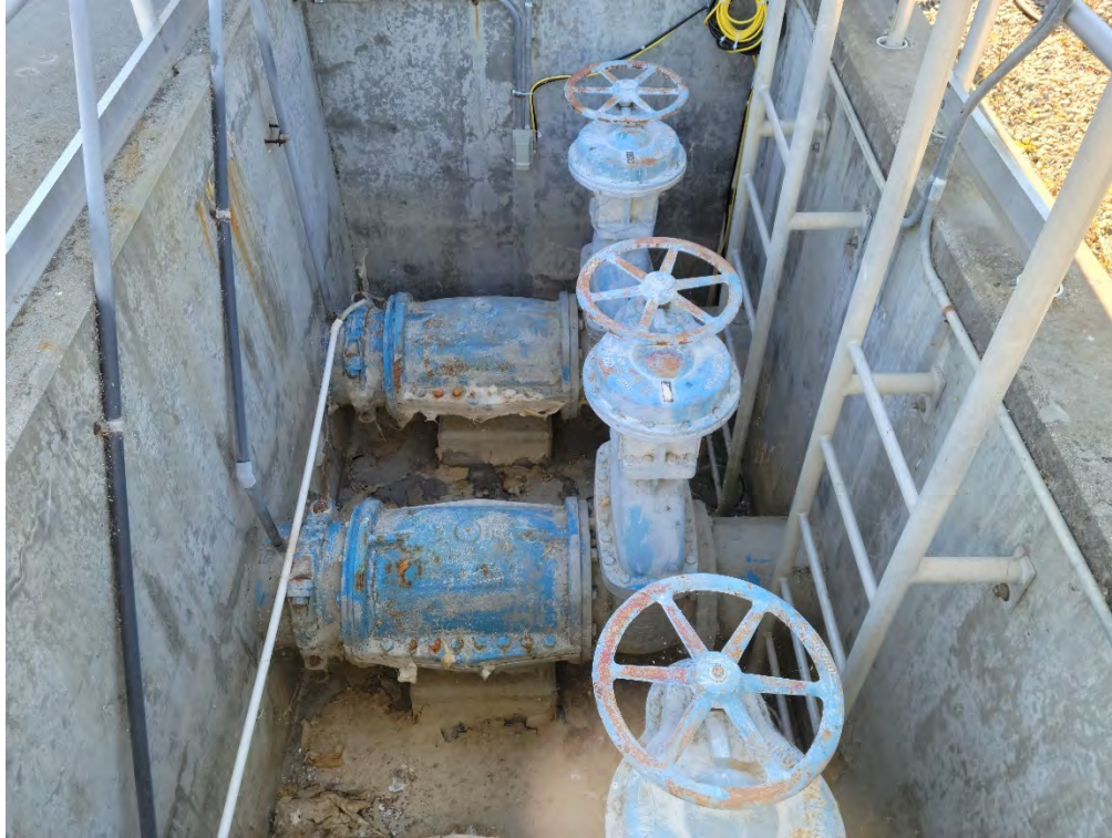
Figure 5 - FERFF Pump Discharge Valves
