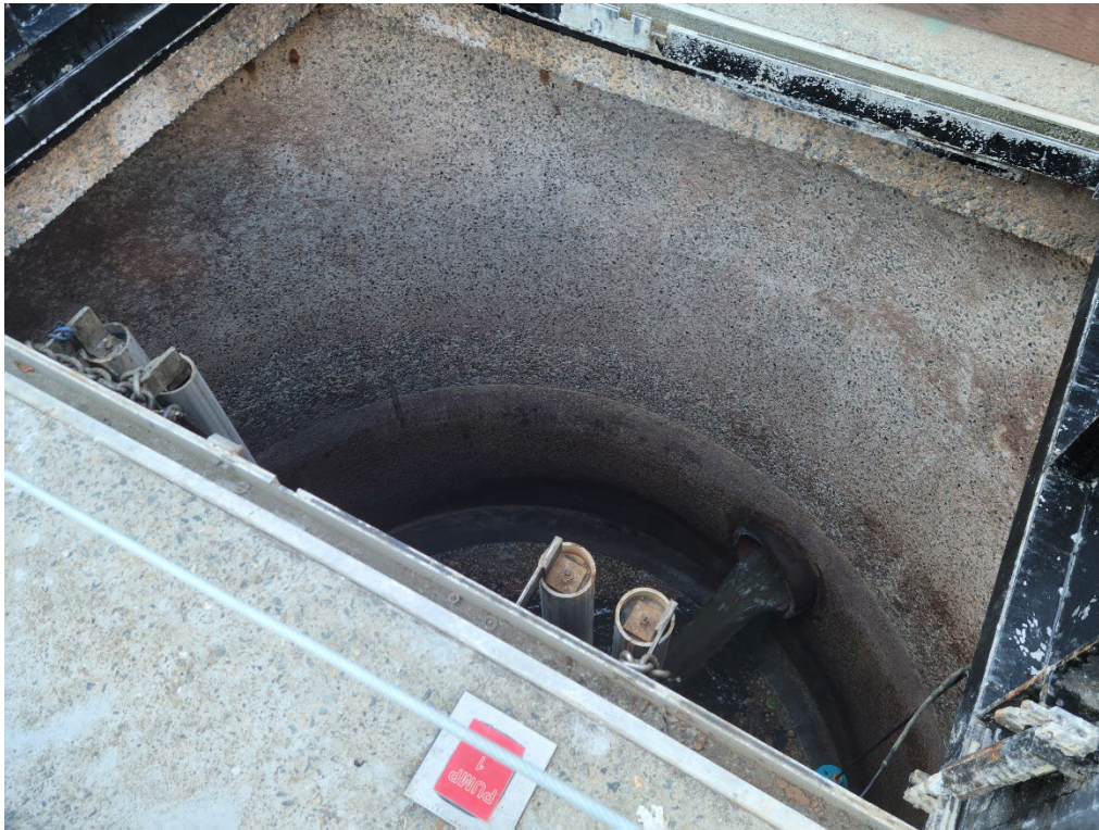
Figure 7.3 Wet Well Corrosion Above Water Surface at Hamilton-Henderson Wet Well Walls
