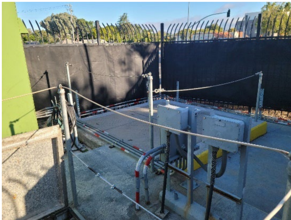
Figure 7.1 Willow Pump Station Wet Well Cover and Equipment
