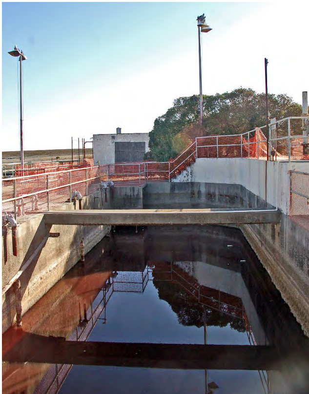
Photo 26. Pre-Treatment Tanks. View looking east.
