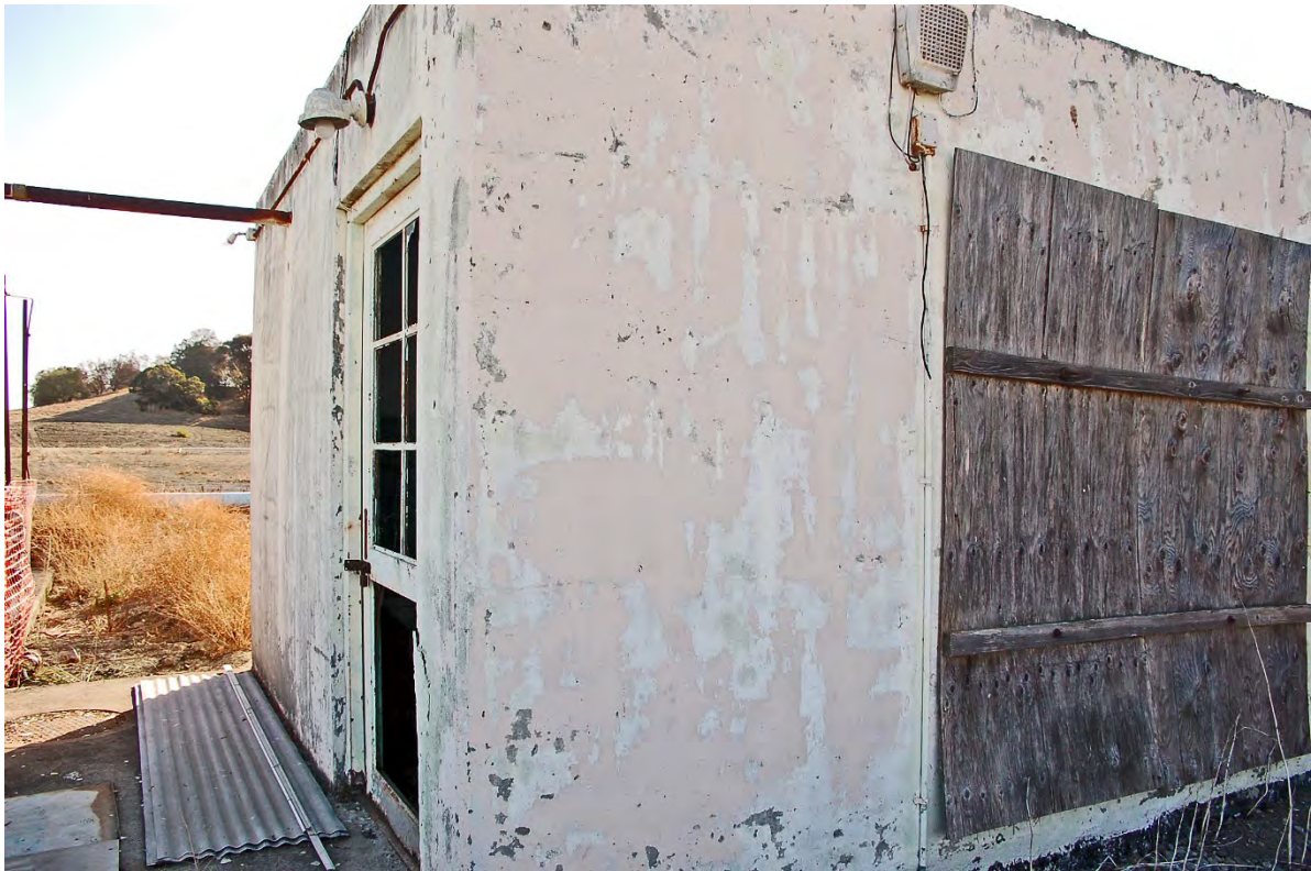
Photo 28. Pump House: View looking southeast.
