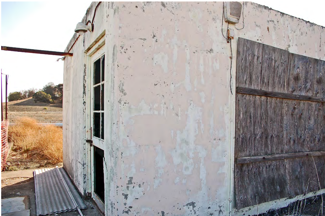
Photo 28. Pump House: View looking southeast.
