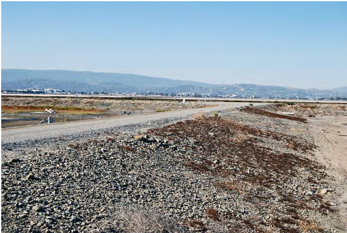
Photo 6. Levee and gravel road between Pond 1 (left) and Pond 2 (right). Typical example of internal earthen berms around ponds and circulation. View looking southwest.
