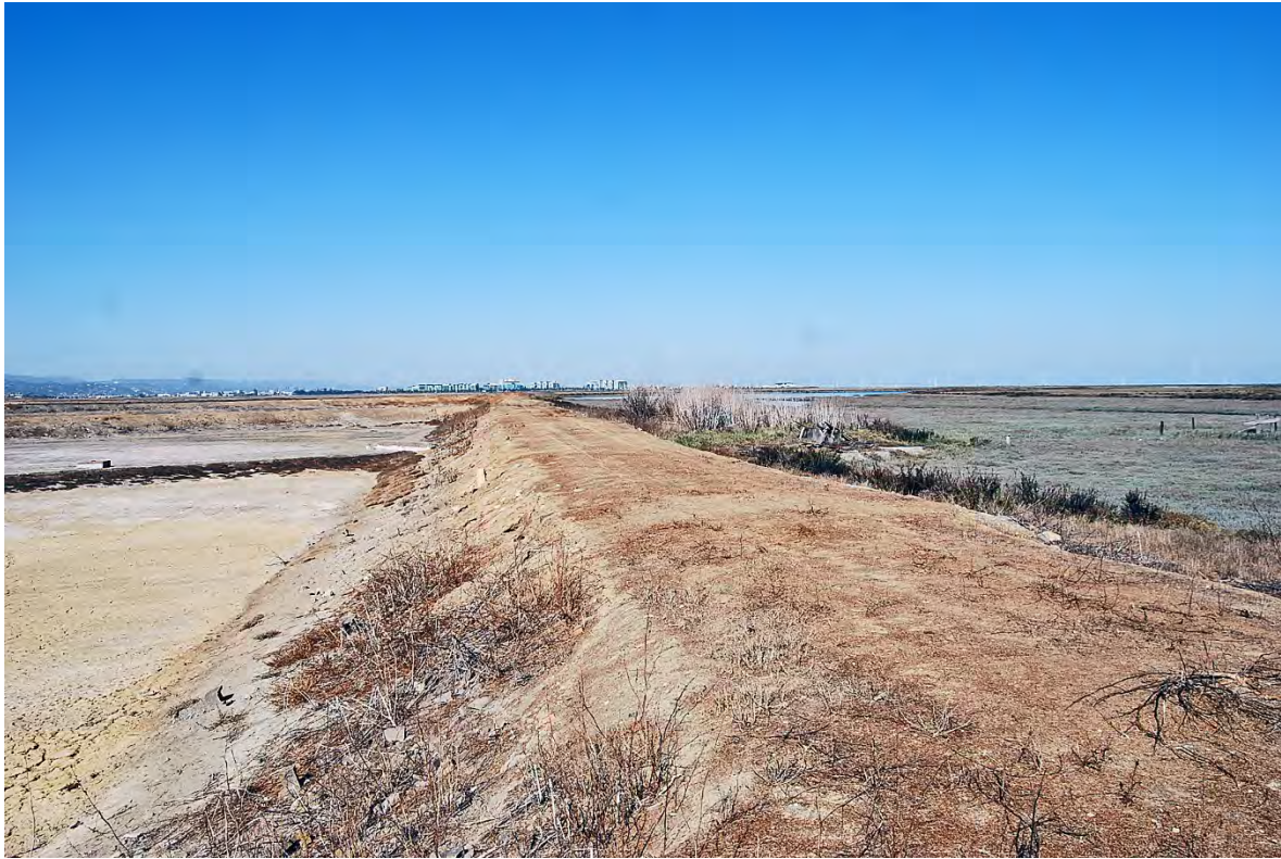
Photo 9. Levee and dirt road along the north side of the property. Pond 3 (left) and Westpoint Slough (right). View looking west.
