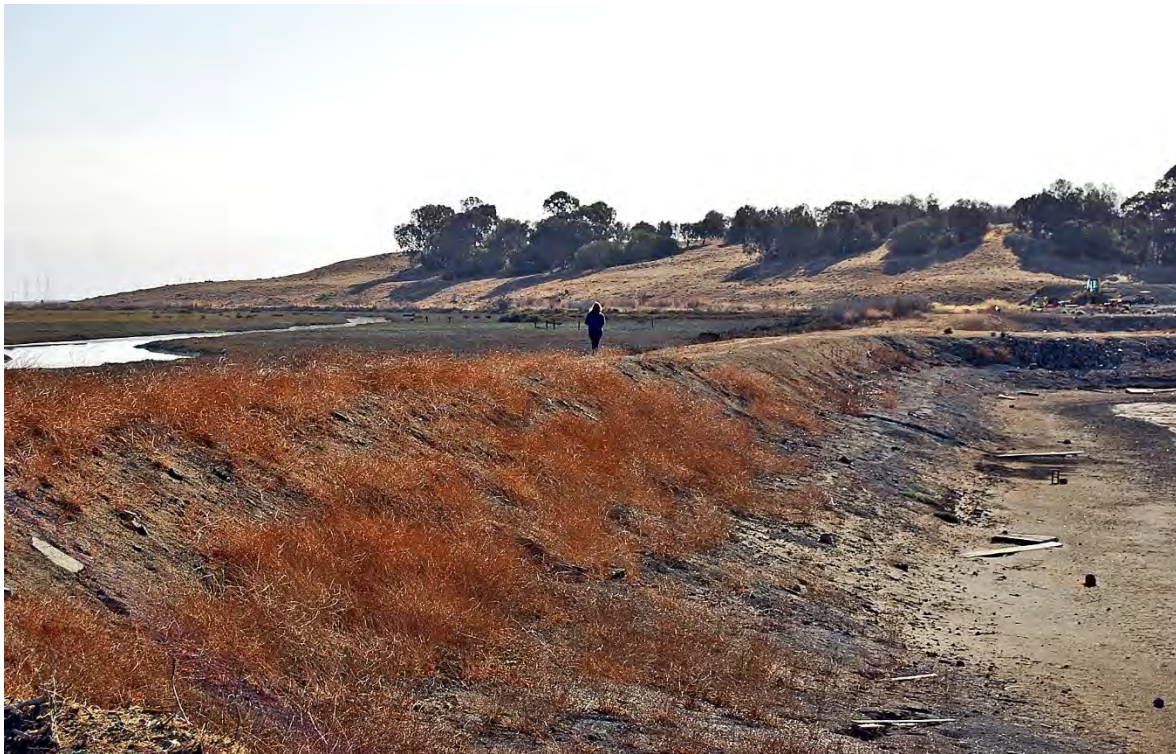
Photo 8. Levee and dirt road along the north side of the FERRF property. Levee provides separates the property from Westpoint Slough (left) and forms the north side of Pond 2 (right foreground) and Pond 3 (right background). View looking east.
