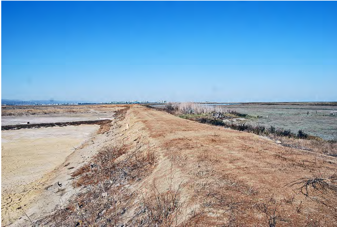
Photo 9. Levee and dirt road along the north side of the property. Pond 3 (left) and Westpoint Slough (right). View looking west.
