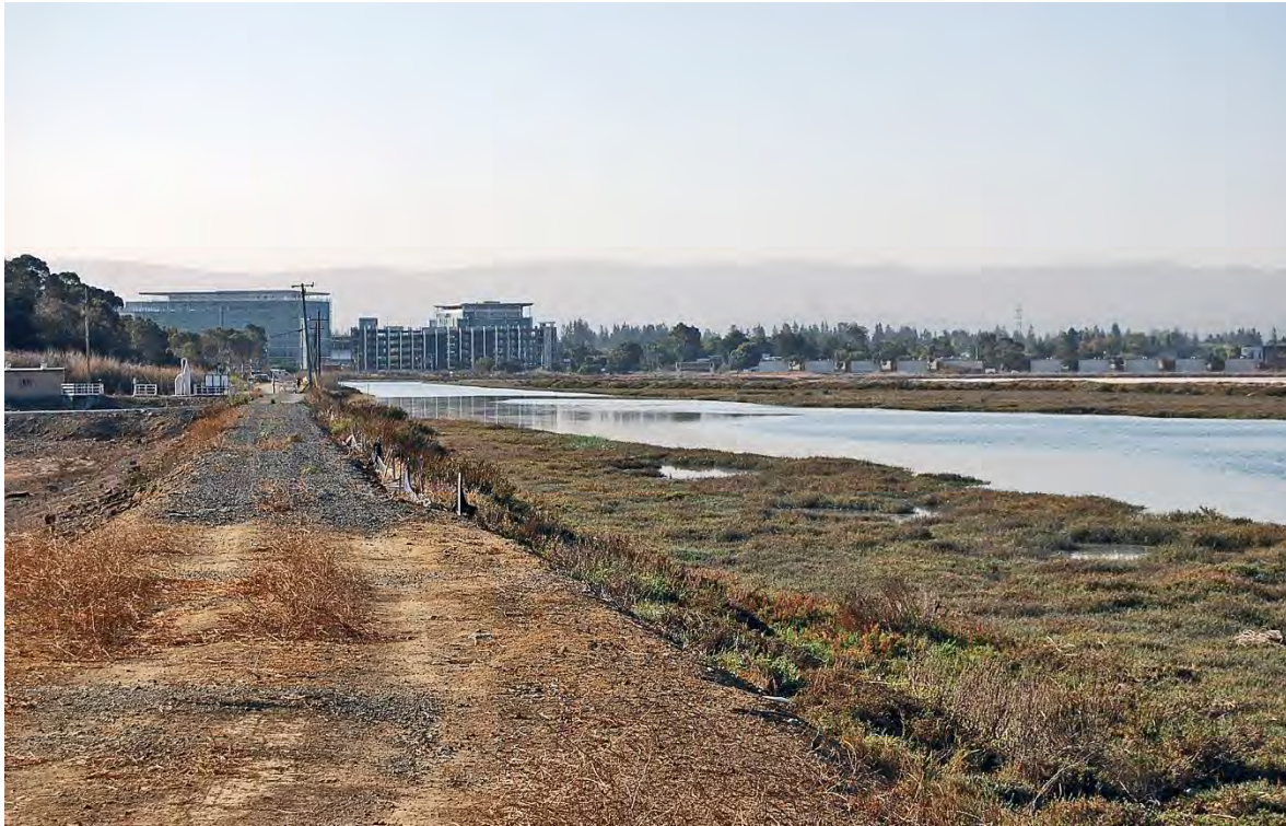
Photo 7. Levee and gravel/dirt road along the west side of FERRF property. Levee separates the property from Flood Slough (right) and forms the west side of Ponds 1 and 2 (left). View looking south.
