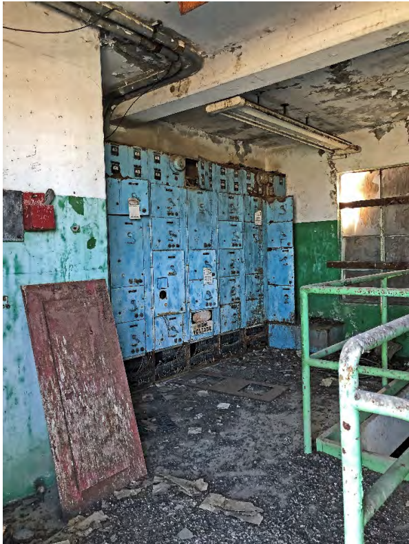
Photo 29. Pump House. Interior view.
