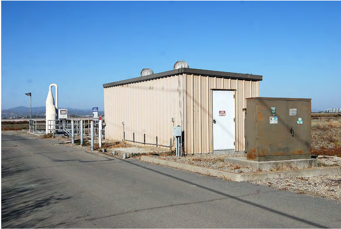
Photo 3. Return pump station. View looking northwest.
