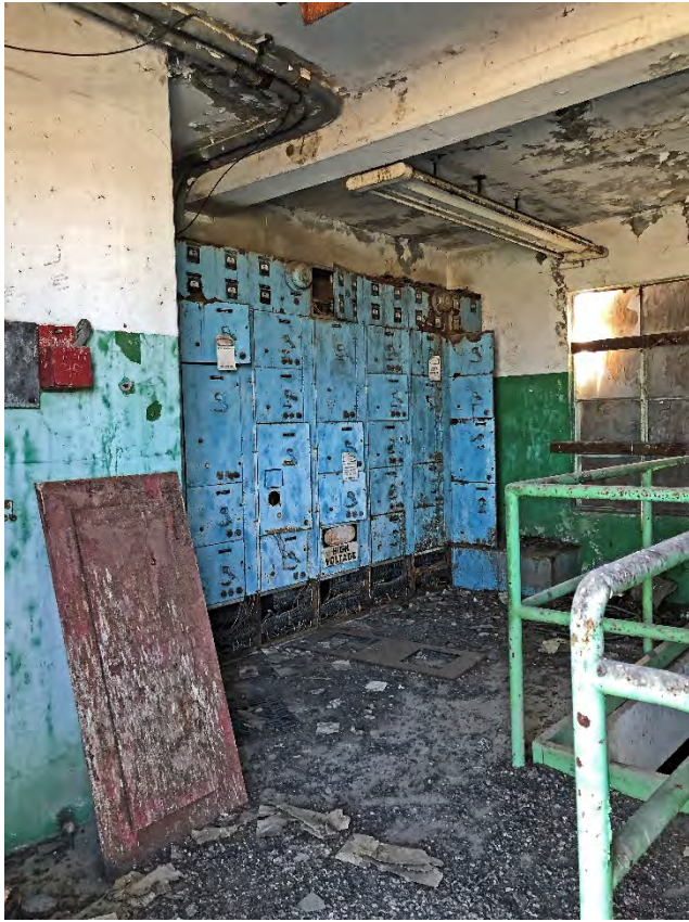
Photo 29. Pump House. Interior view.
