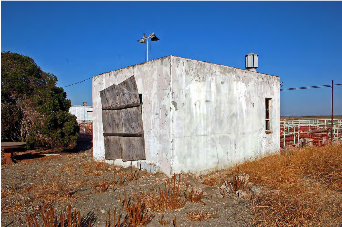
Photo 27. Pump House: View looking northwest.
