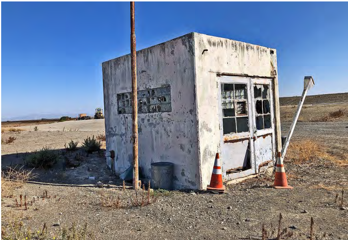
Photo 30. Chlorination Building. View looking northeast.
