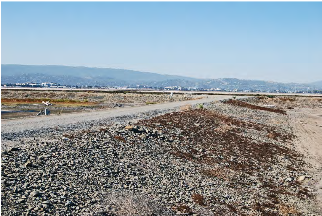
Photo 6. Levee and gravel road between Pond 1 (left) and Pond 2 (right). Typical example of internal earthen berms around ponds and circulation. View looking southwest.
