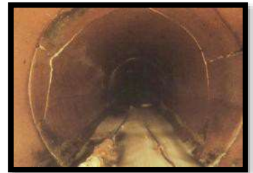
Cracked Clay Sewer Pipe
